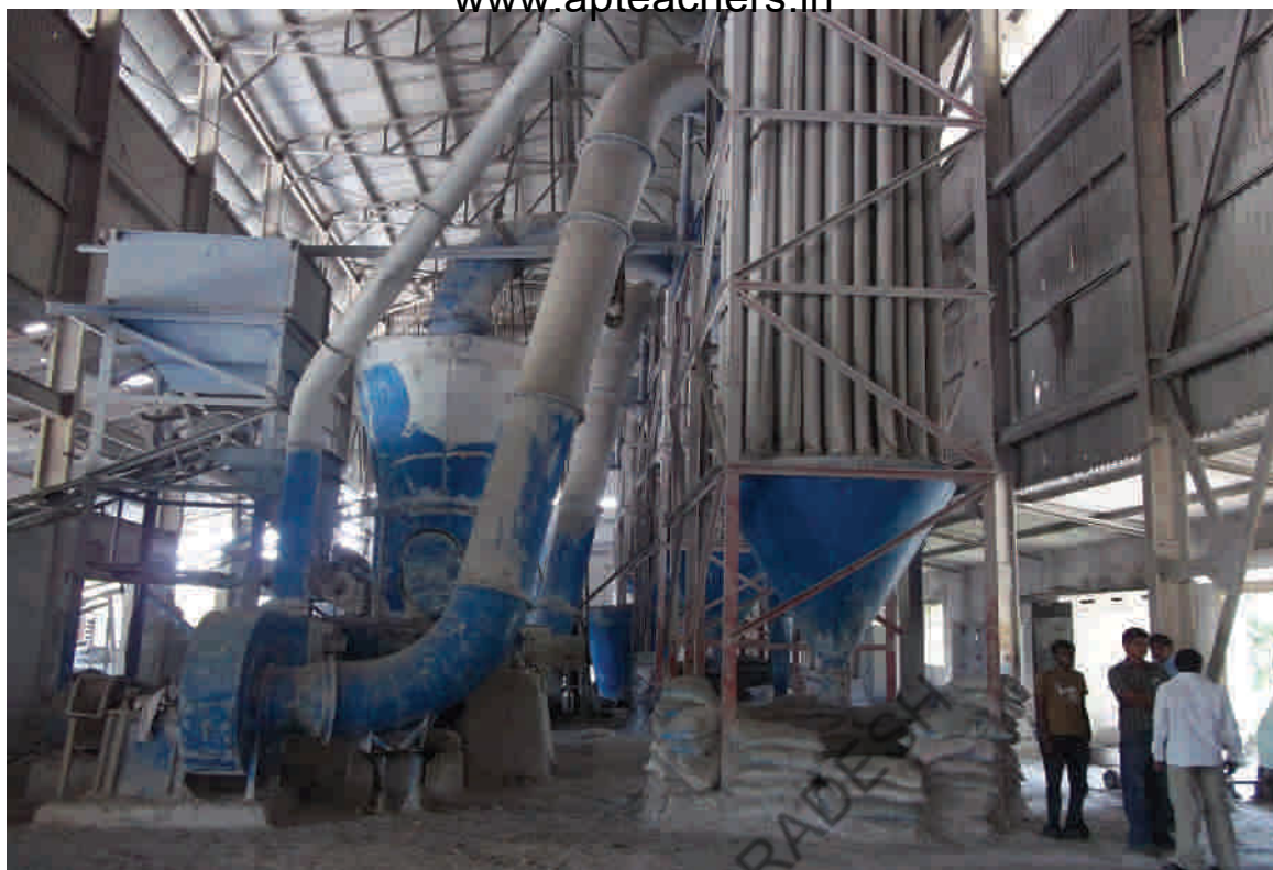
Fig 6.12: Crushing and packing plant
